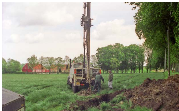
Fig. 2. Field investigations at the Lundeberg locality. Drilling close to the excavated trench.
