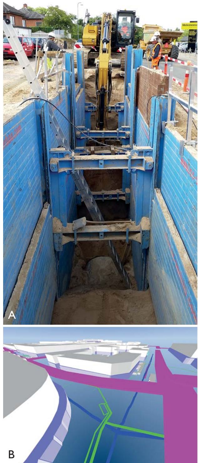
Fig. 3. A: Large sewer in an excavation to be filled with gravel. Image source: VandCenter Syd. B: Anthropogenic model of sewers with other implemented data elements (roads, pipes and buildings).
